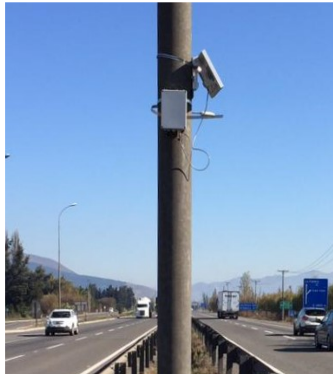
Permanent Median Mount with Solar
